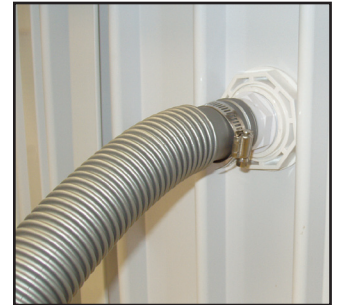
Figure 17 — Free end of hose attached to return
